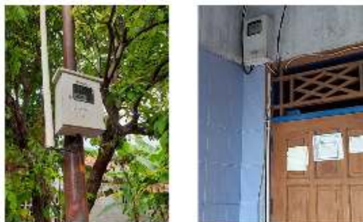
Fig. 6. Cluster and Limiter Systems for Connecting Electricity to Residents' Houses
